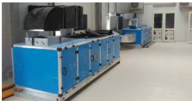
→ Air Handling Unit
